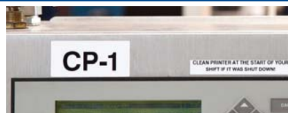
Control Panel & Electrical Panel Labels
